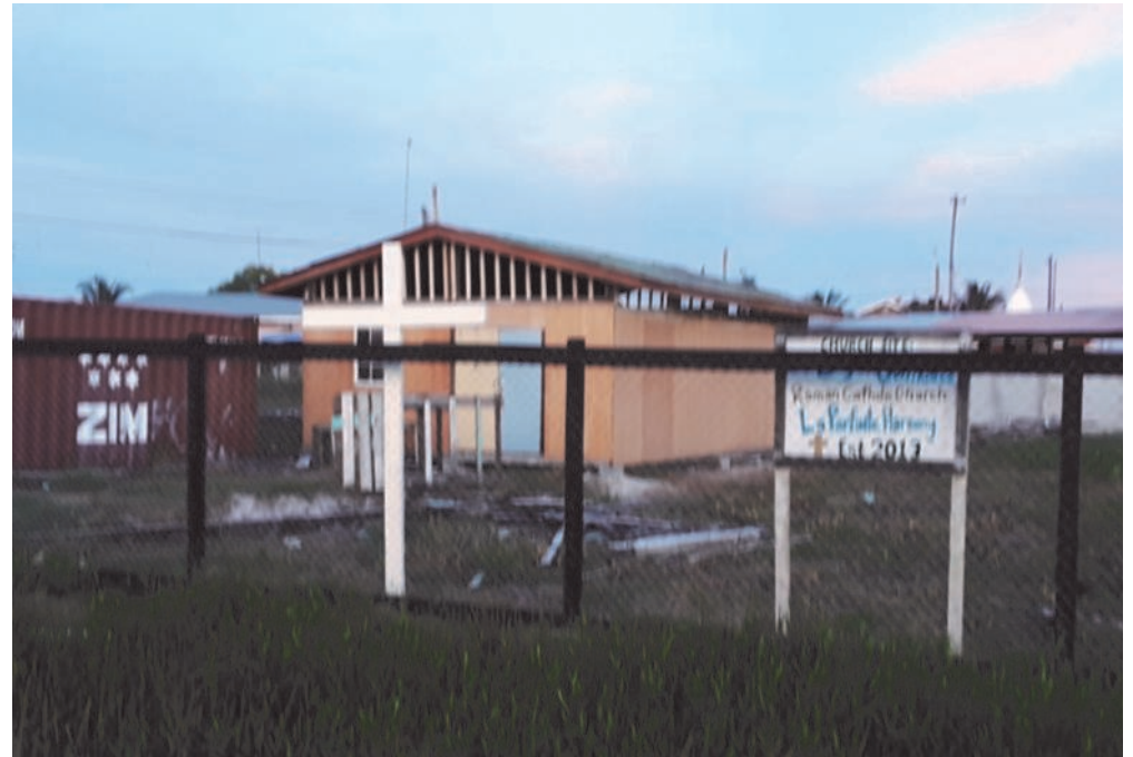
The temporary structure being built at La Parfaite Harmonie for the holding of religious services and other community events.
